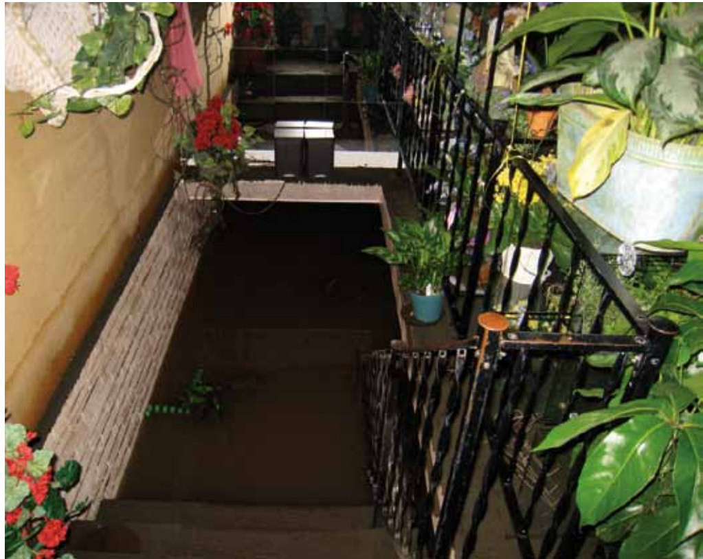
The basement of the shop was completely flooded.
