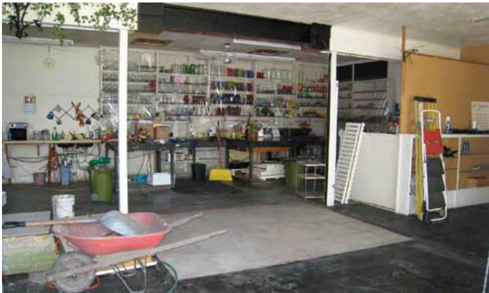
Here, the old cooler has been removed from the center of the shop and the space is waiting to become the new location of the front counter.
